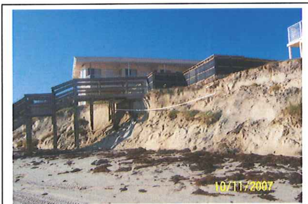
Figure 5: Greatest losses occurred seaward of protruding structures.
