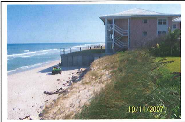
Figure 3: Erosion losses were greatest in front of seawalls and rock revetments.
